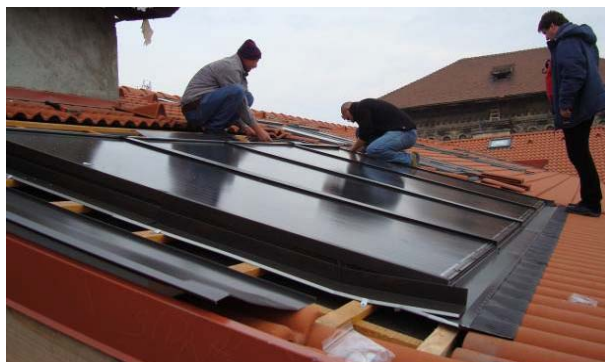
Figure 2. PV modules mounting
