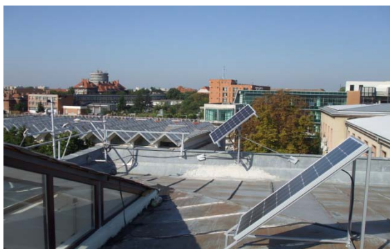
Figure 5. Total view of the PV system on the roof of WUT
