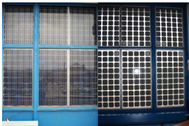
Figure 8. The photovoltaic system at PUB – seen from outside (a), seen from inside (b)
